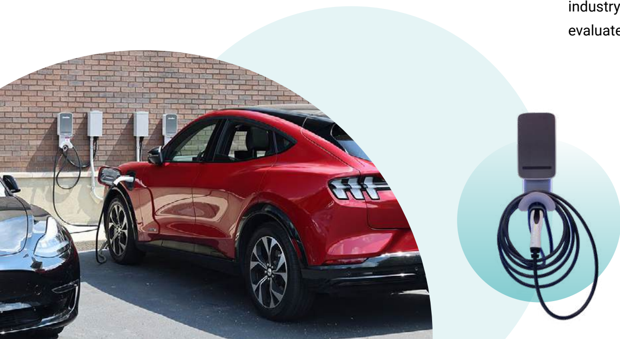
EV Charging Stations at HQ
